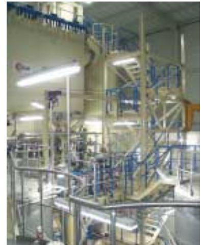
Production plant, GFG 850
