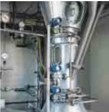
AGT 400, constructed in 1981
